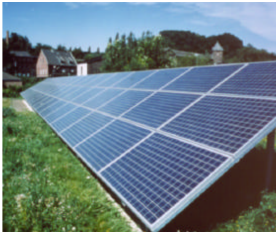
Fig. 1: PV system in Mülheim a.d. Ruhr
